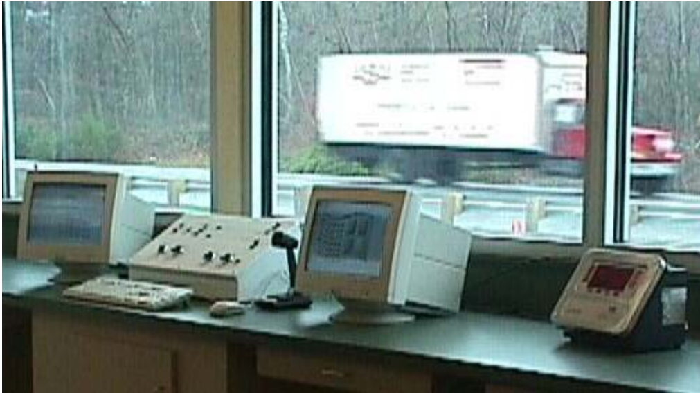
Typical Multi-Scale Weigh Station Instrumentation
